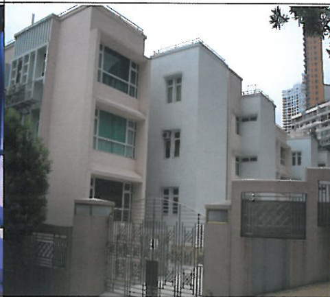
External Wall Renovation and Concrete Repair 大廈外牆翻新改建及石屎維修
